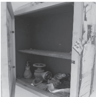
Fig.1 Lack of supporting fire-fighting facilities
